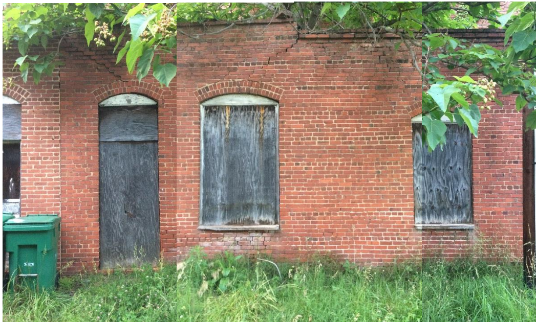
Composite photo showing cracked brick walls requiring steel plate stabilizers.
